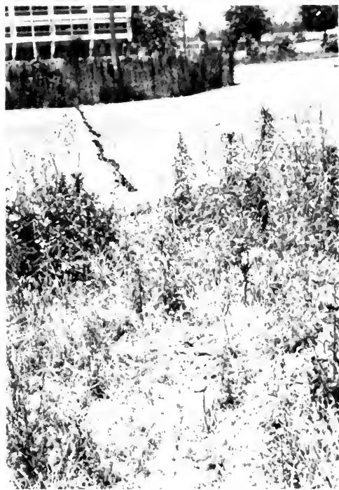
Photo 6. View west-southwest from 75 m (250 feet) east of main building of Olive View Hospital (locality 40). Crack visible in foreground is down on south as much as 1 cm (0.4 inch). Brunton compass for scale.
